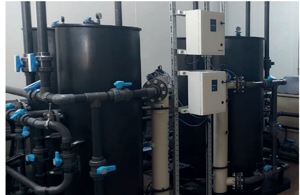
Mechanical Filter Units
